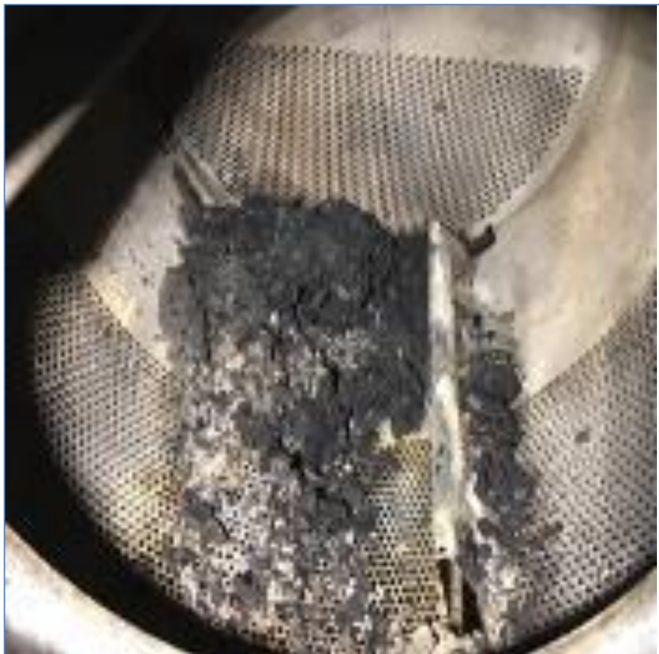
Image 2: Fire damaged contents inside a tumble dryer
