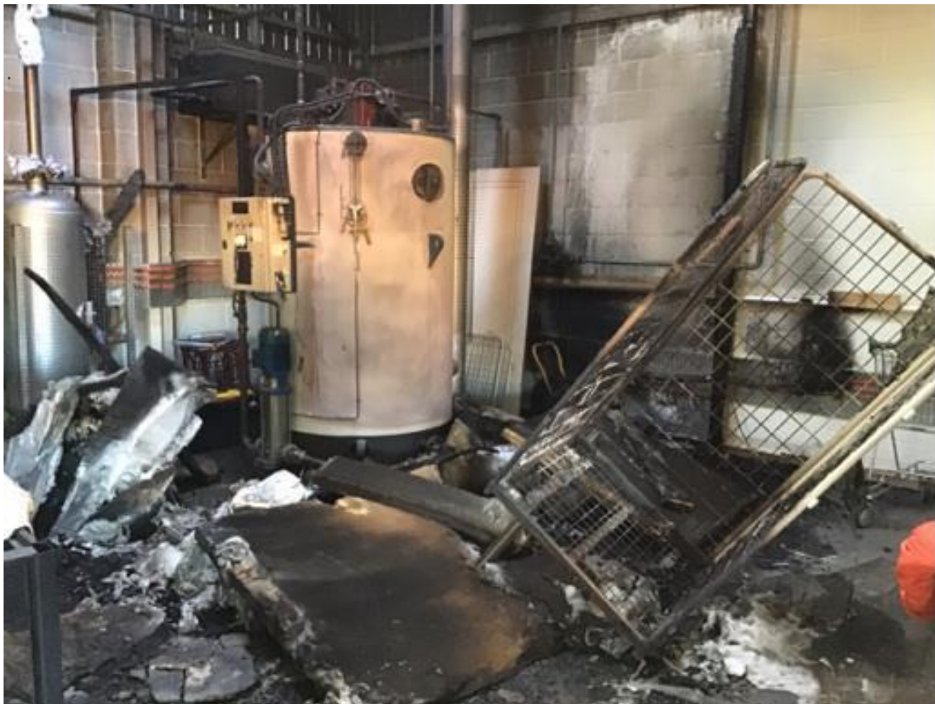
Image 1: Commercial laundry damaged by fire
